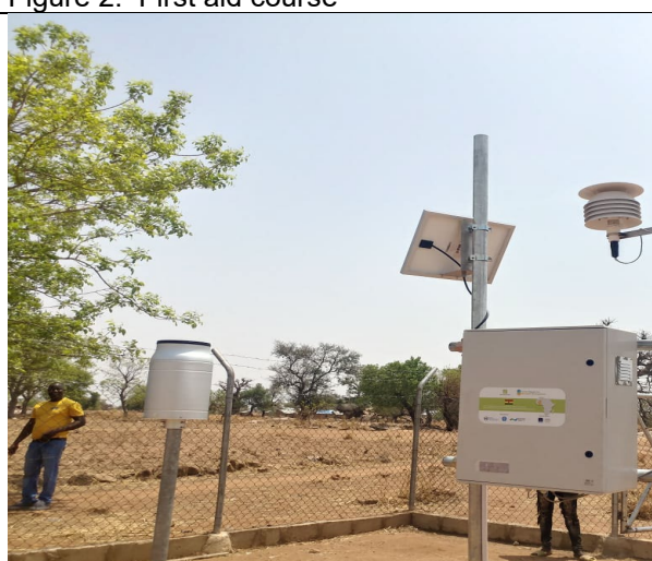
Figure 4: Installed meteorological station
