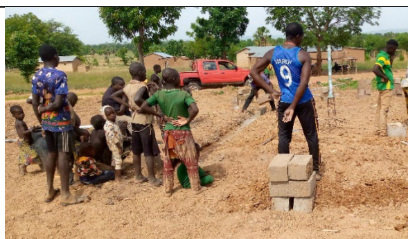
Figure 2: Construction of a basement for the meteo station to be installed in the Tabota community
